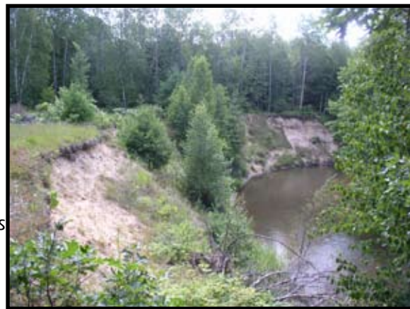
Streambank erosion contributes sediment to the river and needs to be repaired if possible.
